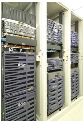
The powerful Sun servers in operation at the Data Center are installed in an easy-to-use rack pre-wired for high-speed network operation.
